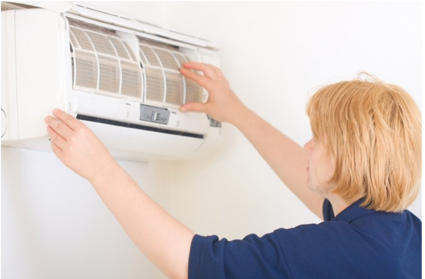
Replacing or cleaning air conditioner filters is a critical maintenance task. | Photo courtesy of ©iStockphoto/firemanYU.
